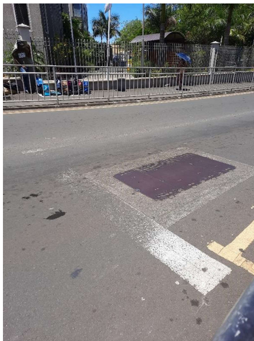
Figure 40: Faded Road Markings in (i) Central Flacq
