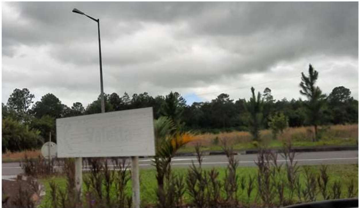
Figure 42: Faded Road Traffic Signs at Valetta
