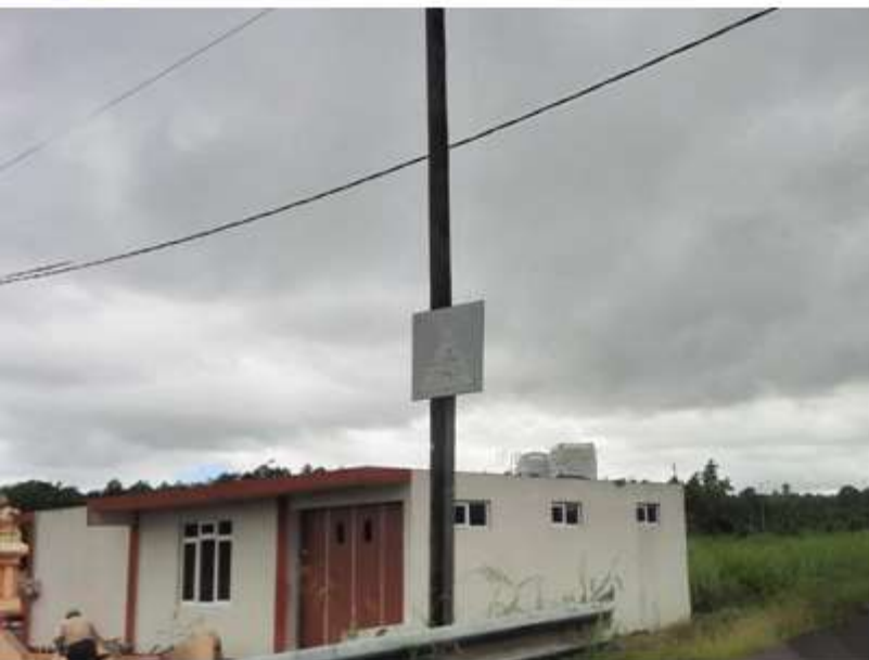
Figure 43: FadedTraffic Signs at Flacq
