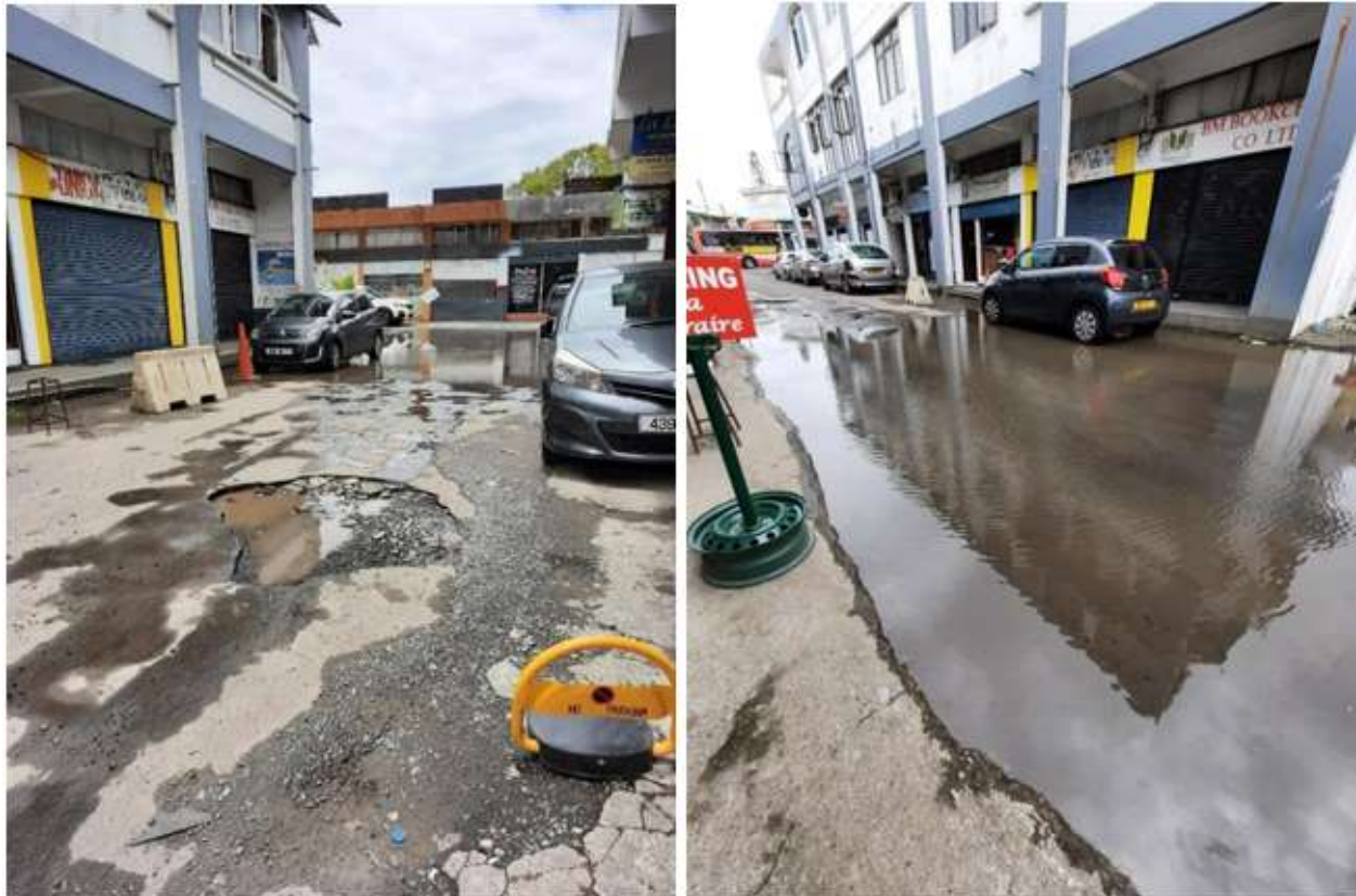
Figure 48: (i) Potholes at Curepipe
